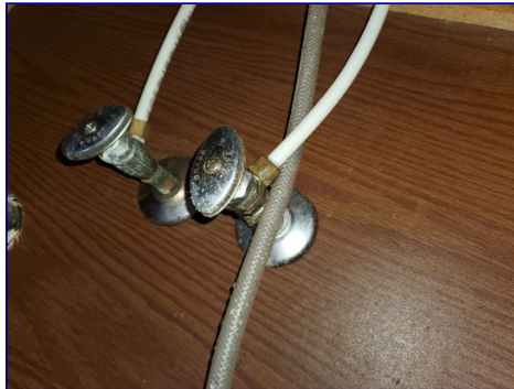
Water supply lines leaking
