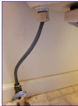
Toilet supply line leaking
