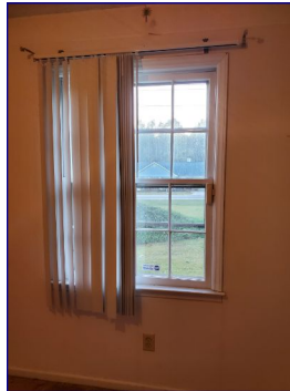
Window would not open
