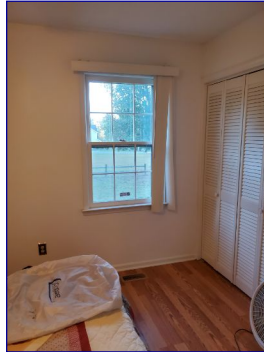
Window would not open
