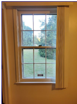
Window would not open
