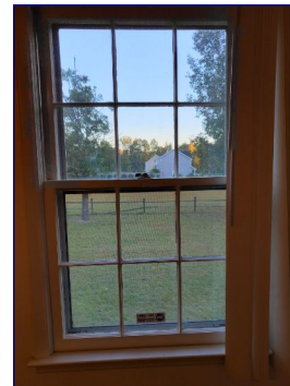
Window would not open
