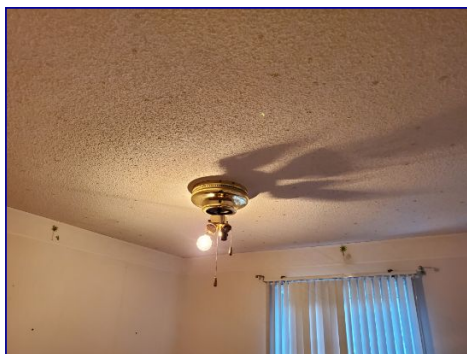
This looks to be what was remaining of a ceiling fan.
