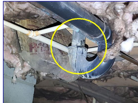
Leak found on this drain pipe
