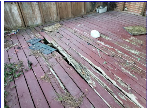
Deck floor is rotted
