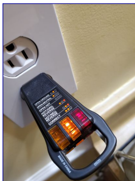
Electrical receptacle showed reverse polarity. Left of sink.
