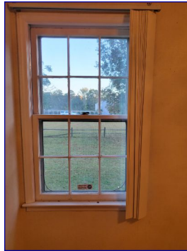
Window would not open
