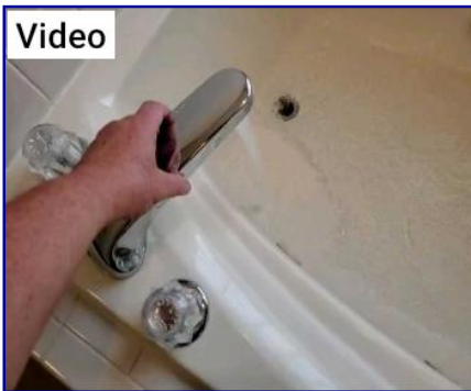
Bathtub faucet loose.
